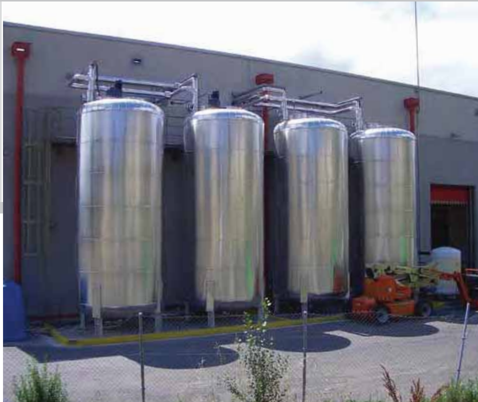
PU-Rohstoff-Tanklager PU raw material tank storage
